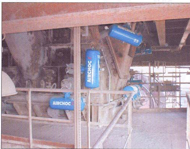
Figure 1. AIRCHOC® on preheater.
