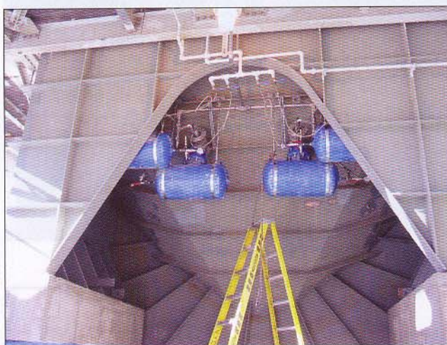
Figure 4. Kiln inlet with AIRCHOC®.
